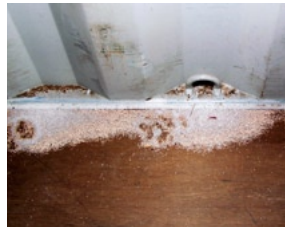
Plastic granulate on or between floor joints.
