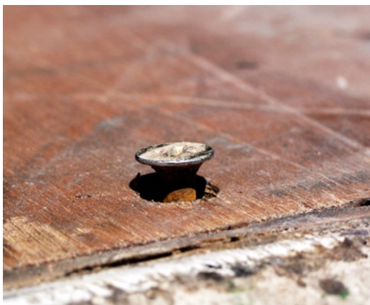
Protruding floor screws
