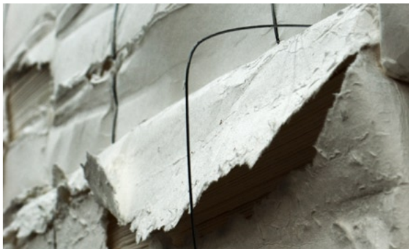
...and damaged wrapping
