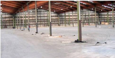
Accumulated debris around pillars
